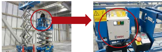
Example installation of the trapping prevention system
